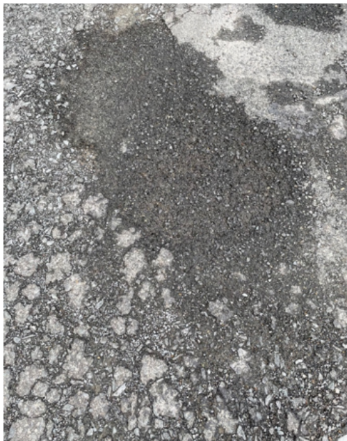
Improperly repaired potholes
